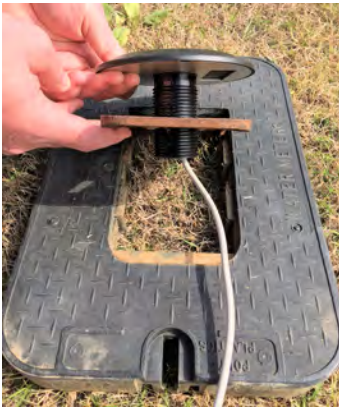
Figure 28 – Antenna and Pit Lid
