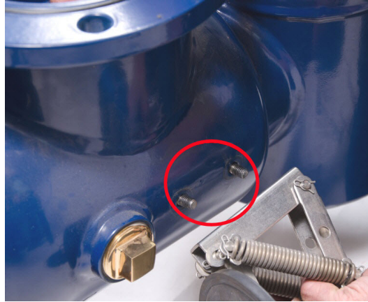
Figure 45 – Knuckle Valve Bolt Holes
