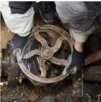
Figure 16 Isolation Valve - Downstream of the Meter Under Test
