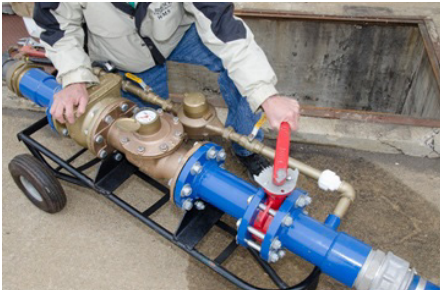
Figure 7 Purge Air from Test Setup
