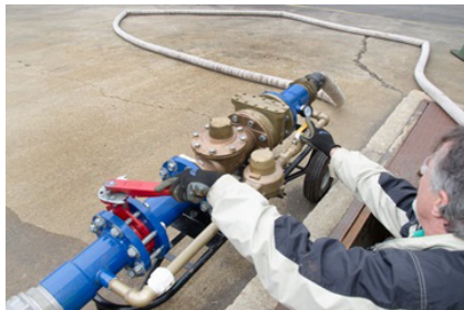
Figure 15 High Side Valve on Reference Meter
