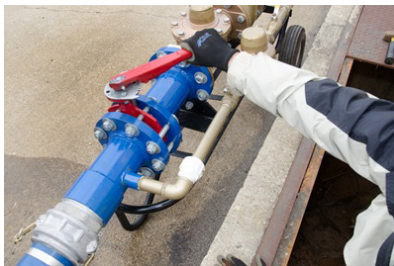
Figure 11 Back-Flushing the Meter
