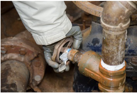
Figure 14 Test Riser Valve Attached to Meter Under Test
