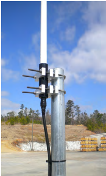
Figure 78 – RF Antenna to Mast
