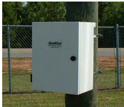
Figure 54 – Mounted Battery Box
