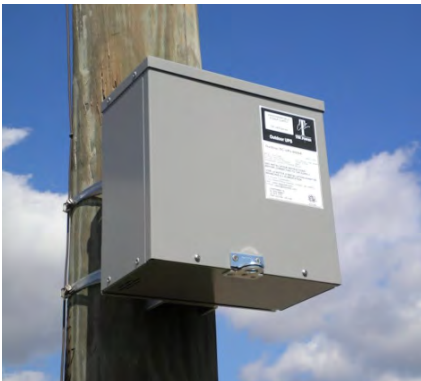
Figure 61 – UPS Attached to a Large Pole
