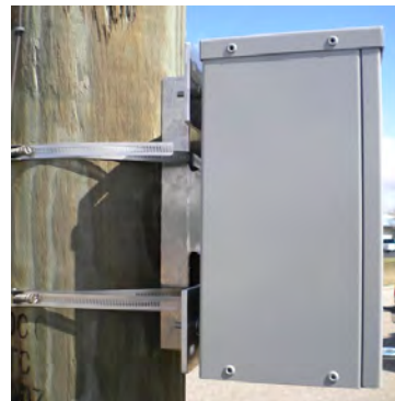
Figure 62 – UPS Attached with Clamps
