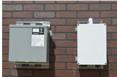
Figure 65 – UPS Mounted on a Wall
