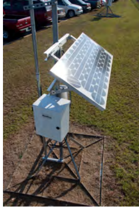
Figure 31 – Gateway Solar Panel
