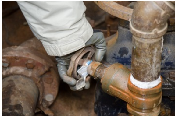
Figure 17 – Test Riser Valve Attached to Meter Under Test
