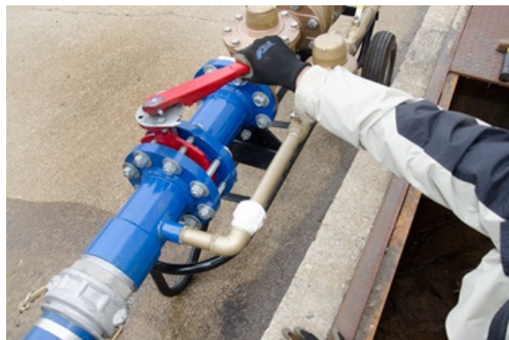
Figure 14 – Back-Flushing the Meter
