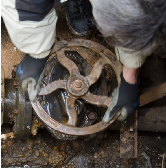
Figure 19 – Isolation Valve - Downstream of Meter Under Test
